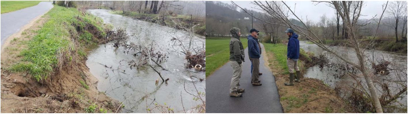
(Left) This bank failure caused by a fallen tree threatened the existing greenway. (Right) Watauga County meets with Adam Williams, Brushy Fork Environmental Consulting.
