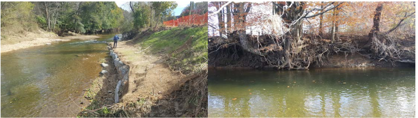
(Left) Rock structure paid for by Watauga County to stabilize the previously pictured bank failure. (Right) 10 - 15 foot vertical banks.
