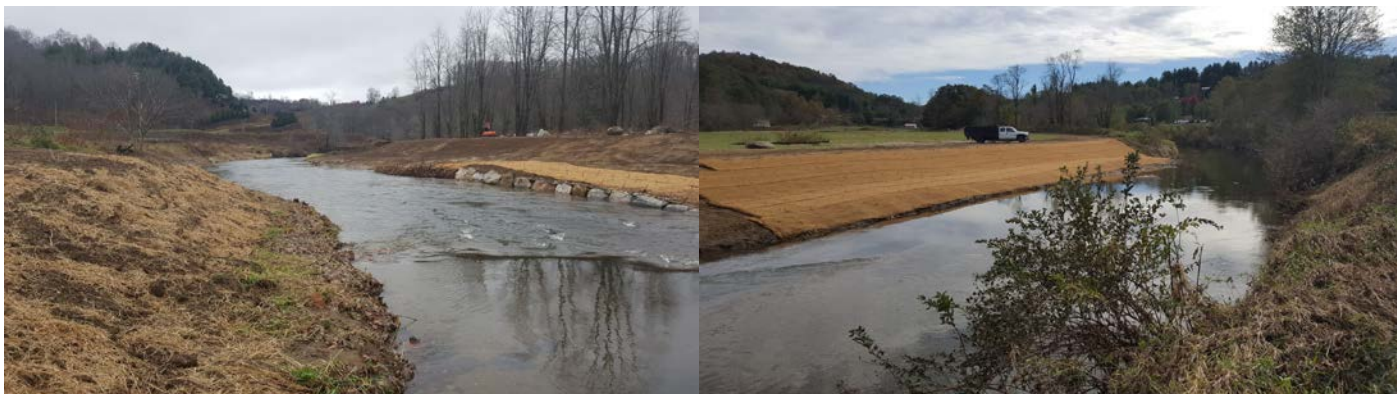
(Left) Flood benches to provide a floodway, and rock structures to stabilize the banks during construction. (Right) Bank sloping, coconut fiber matting, and native woody plant installation during construction.
